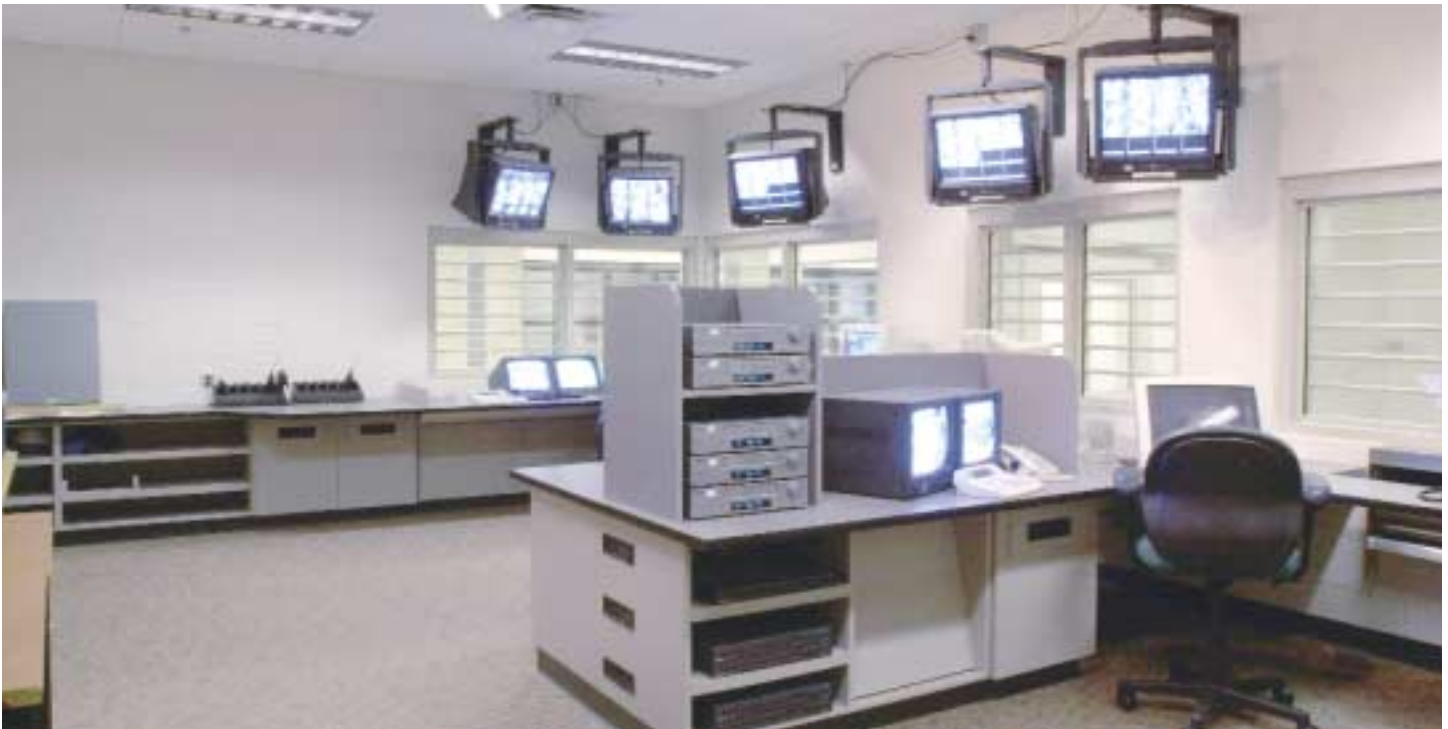
Each operator station can automatically control and call up any camera based on events such as intercom calls and duress and door alarms. The system also provides additional safeguards, such as video visitation, which allows inmates to communicate with visitors within a secure area.
